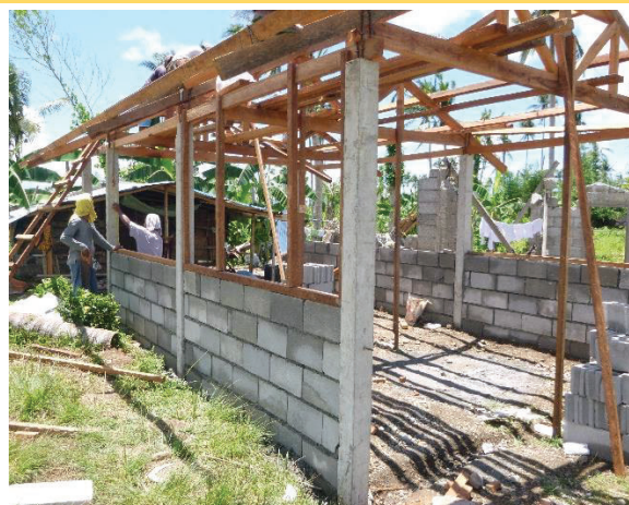
Figure 1: Concrete blocks have been installed between the reinforced concrete columns, up to the level of the window sill of this core shelter in Tabontabon, Leyte. Credit: Philippines Red Cross Haiyan Shelter Programme (Photo W. Eastwood)
